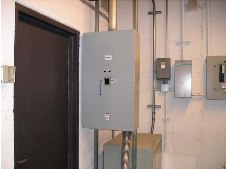
Photo 7: Main electrical service equipment
