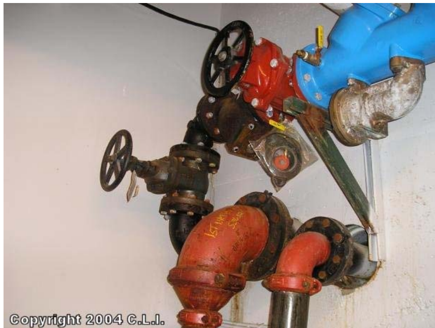
Photo 2: Main domestic water service entrance
