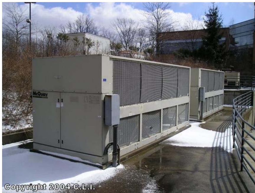
Photo 4: Main air conditioning equipment
