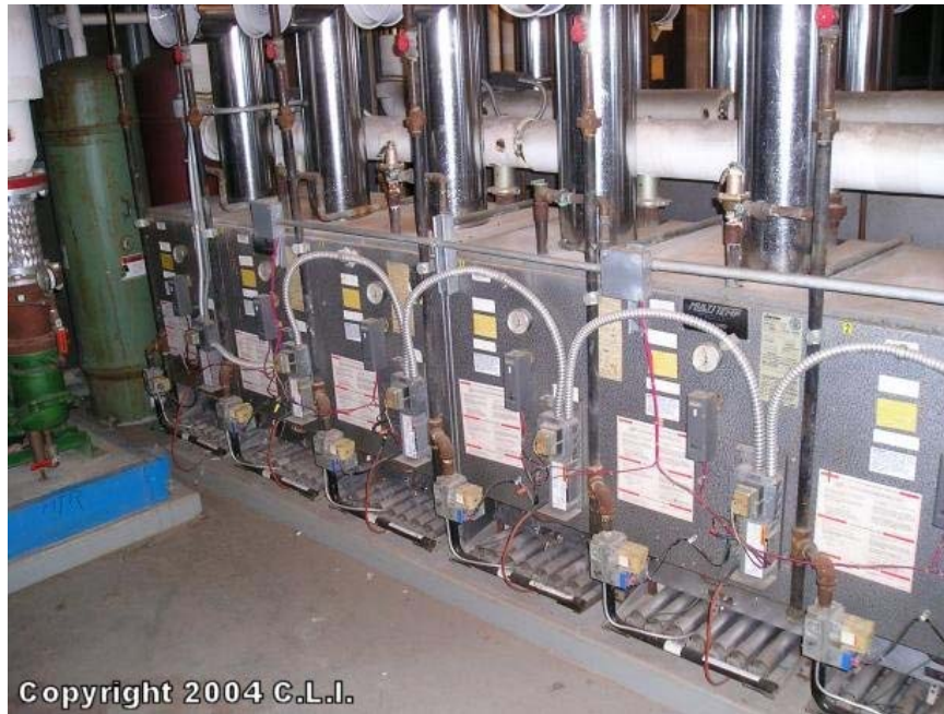
Photo 3: Main heating equipment
