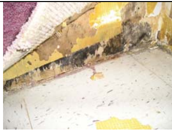
Figure 1 Damage behind carpeted walls
