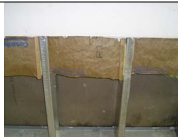
Figure 4 Steel stud, batt insulation, water damage
