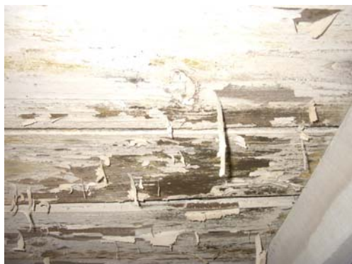
Figure 1 – (Before) Poor mold remediation project.
