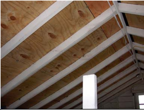
Figure 2 – (After) Two Yr. after correcting building issues
