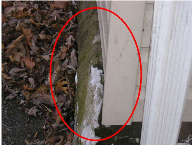
Foundation at rear, drive side of structure indicates bowing/movement of foundation.
