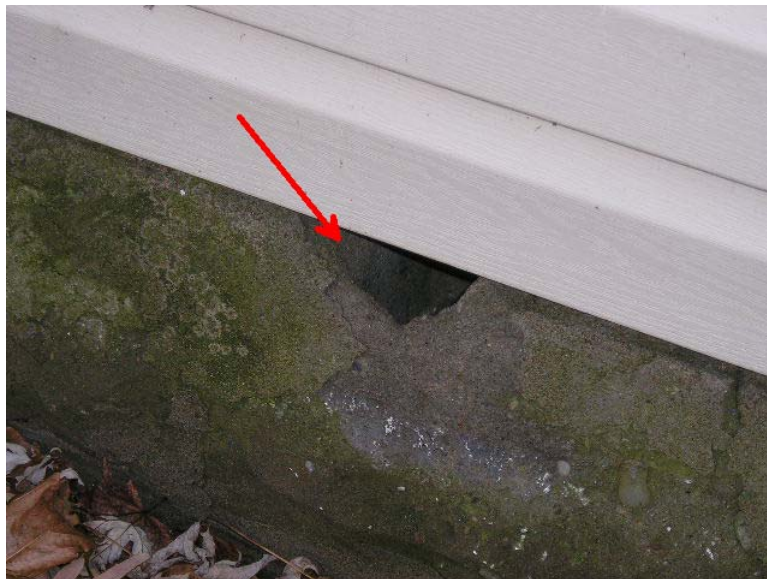
Pointer shows area of foundation at rear, drive side corner which is damaged due to movement and/or moisture.
