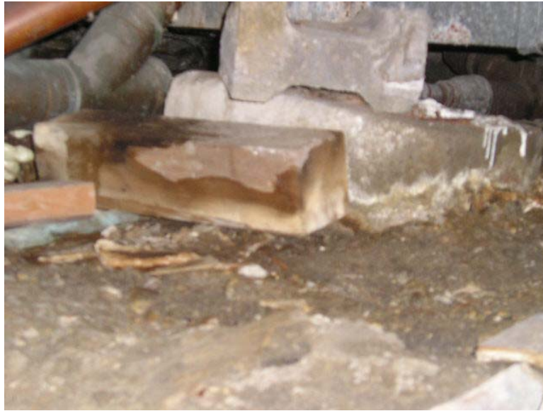
More debris and damaged piers in crawlspace.
