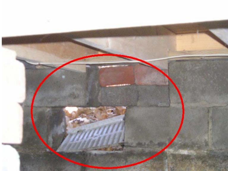
Daylight is visible through foundation walls in various locations throughout the crawlspace. The missing vent shows exterior grade which is higher than vent and is directing water directly into the crawlspace.
